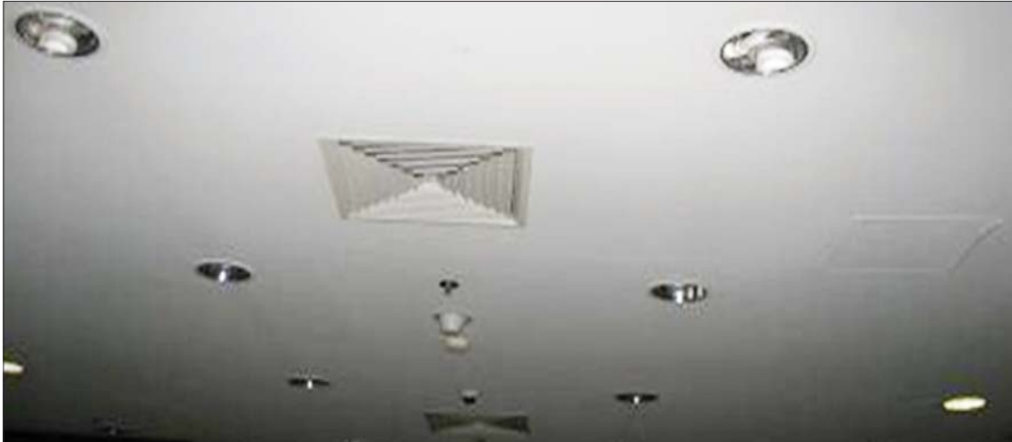
Figure 52. Lobby lighting with compact lamps
